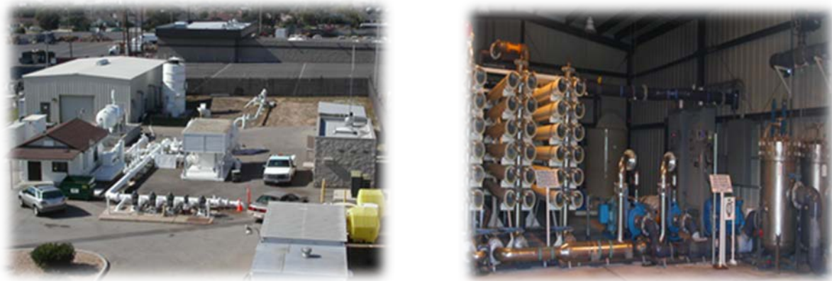
Figure 10-7: Brewer Desalter Treatment Facility
