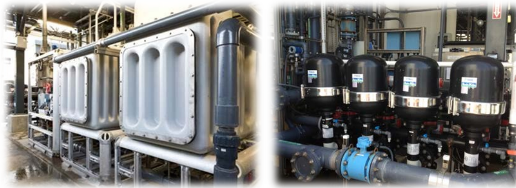
Figure 10-3: West Basin's Ocean Water Desalination Demonstration Facility
