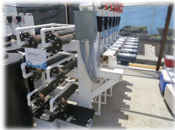
Figure 10-4: Pipe Loop Set Up
