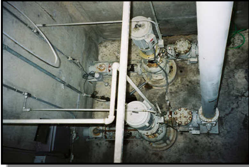
Fig. 6-2. PUMP STATION NO. 1 DRY WELL
