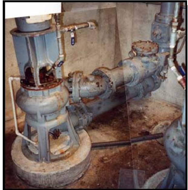
Fig. 6-12. PUMP STATION NO. 9 Dry Well Pump No. 2 and Discharge Piping
