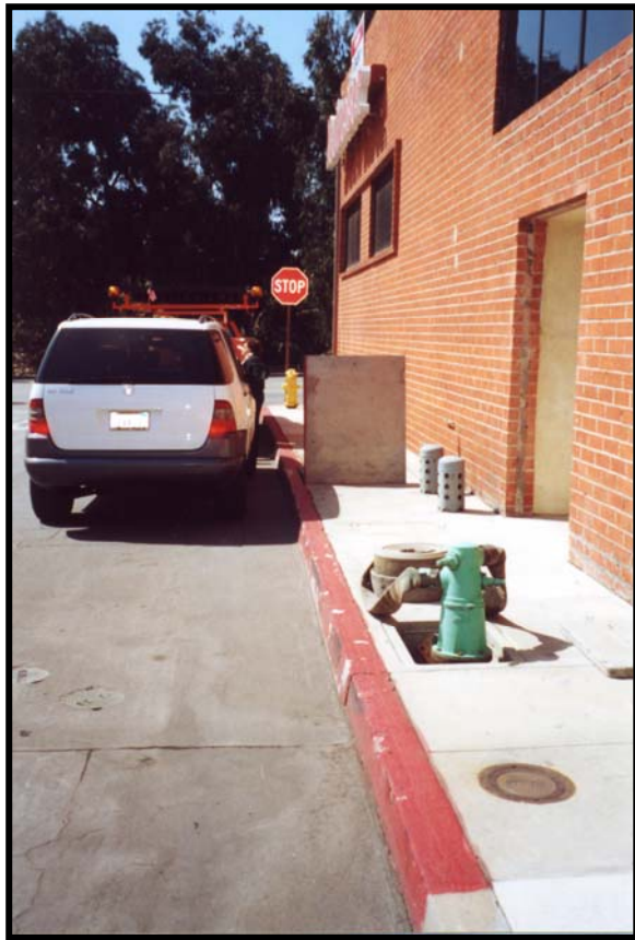
Fig. 6-11. PUMP STATION NO. 9 SITE In Kansas Street North of El Segundo Blvd
