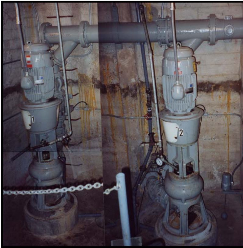
Fig. 6-4 PUMP STATION NO. 2 DRY WELL
