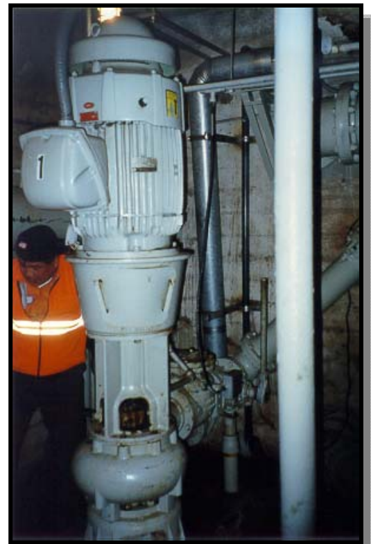
Fig. 6-7. PUMP STATION NO. 7 DRY WELL
