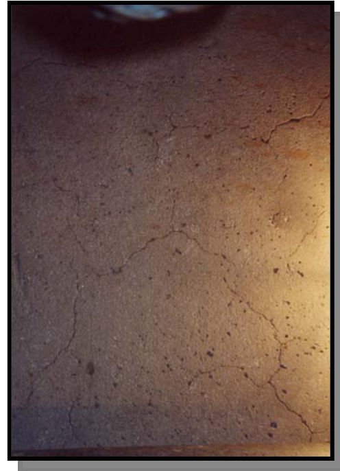
Fig. 6-10. PUMP STATION NO. 8 Dry Well Wall Cracks
