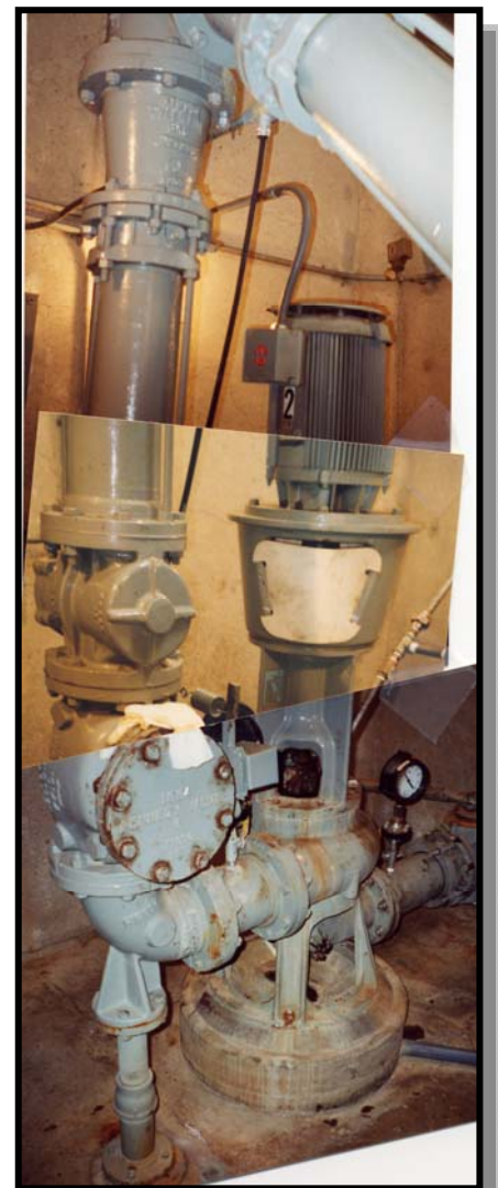
Fig. 6-9. PUMP STATION NO. 8 Pump No. 2 Suction and Discharge Piping
