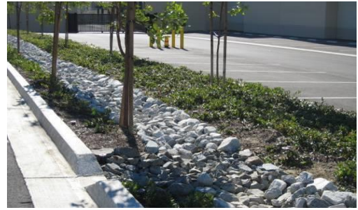
On-site storm water capture system
