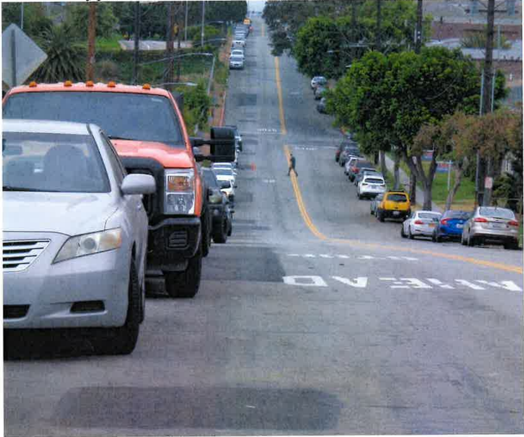
Before: Utility patches on north side of E. Imperial Ave. from McCarthy Ct. to California St.
