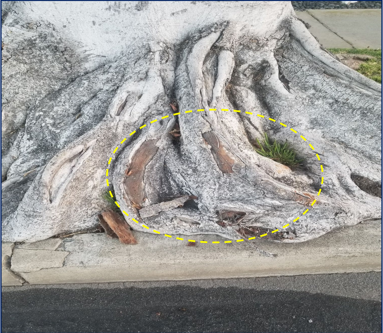
Image 5. Showing the buttress along the curb edge, note the bark is peeling from the top portions.
