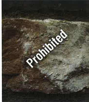
Unnatural looking stone from a worn out mold with poor detailing
