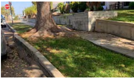
Figure 2 – 536/540 Arena Street damaged asphalt, curb, and sidewalk due to tree roots.
