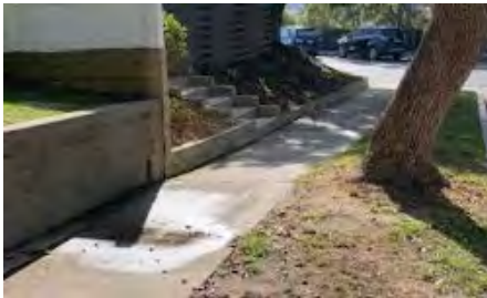
Figure 1 – 506 Arena Street uneven sidewalk and ponding due to tree root uplift
