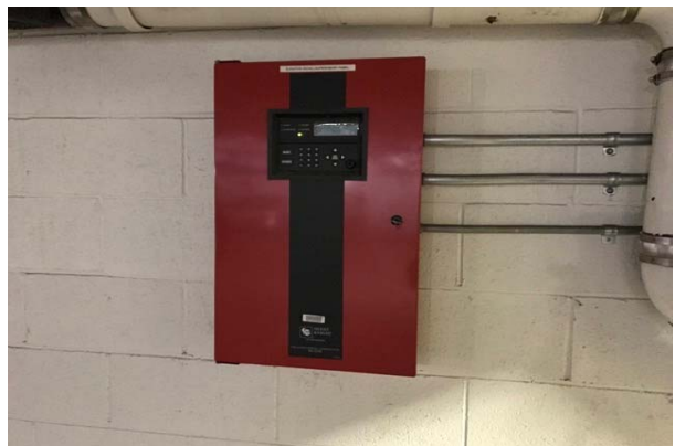
#30 FIRE ALARM CONTROL PANEL
