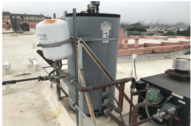
#28 WATER STORAGE TANK
