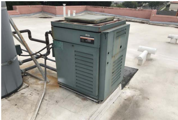
#27 DOMESTIC WATER BOILER
