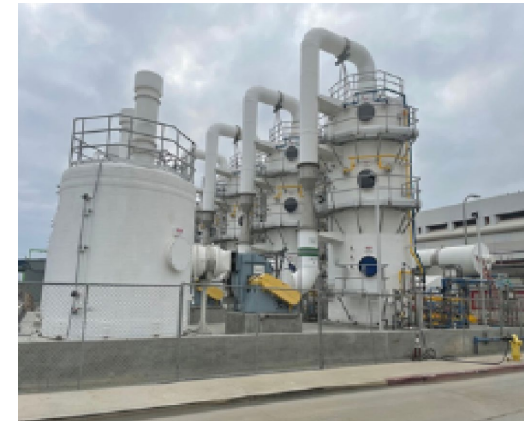
Intermediate Pumping Station BTF
