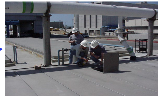
REPLACE TANK COVERS
