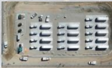
20 MW Battery Storage
