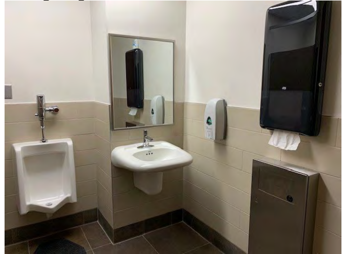
New urinal, urinal cleanout, ADA stall, sink, mirror, paper towel dispenser, waste receptacle, tile, lighting, fixtures, and accessories installed.
